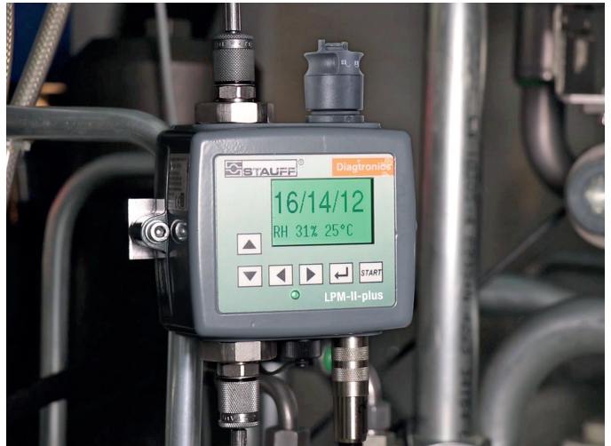
LPM-II-plus in stationary application
